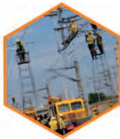
Electric power system
